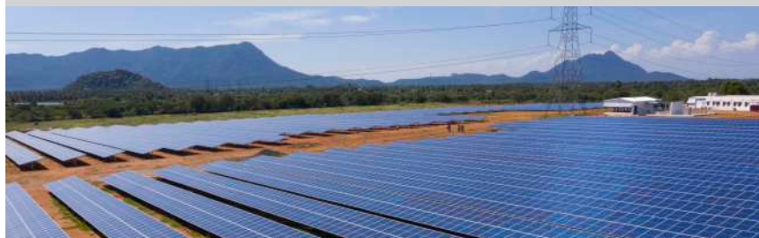
Dollar's solar power plant
