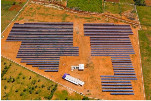
SOLAR POWER PLANT
